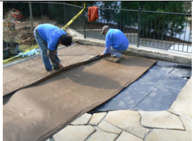
Installation of J-DRain GRS on top of tapered insulation and layer of EPDM.
